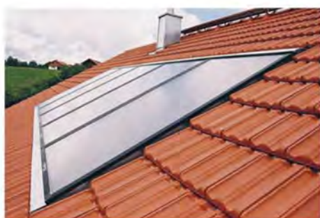
Solar hot water - integrated flat plate collector
